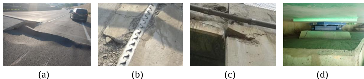
Figure 1 Examples of failures at road bridge expansion joints: (a) Blow-up in road pavement, (b) Lack of joint gap in expansion joint, (c) Failure to wing wall of bridge abutment, and (d) Failures by excessive bridge support movement.
